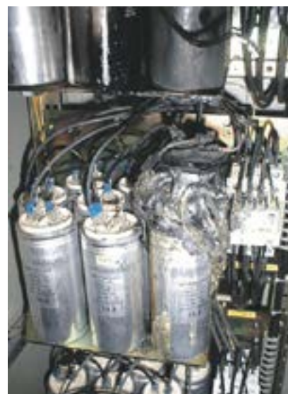
Fig.: Capacitors destroyed by harmonics current
