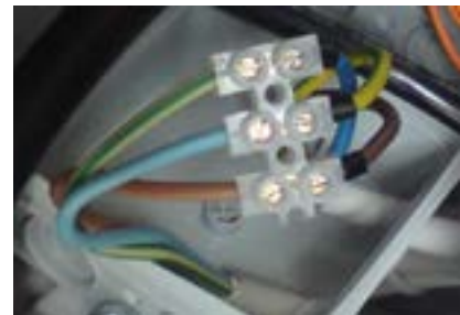
Fig. 7: Here N and PE have been reversed
