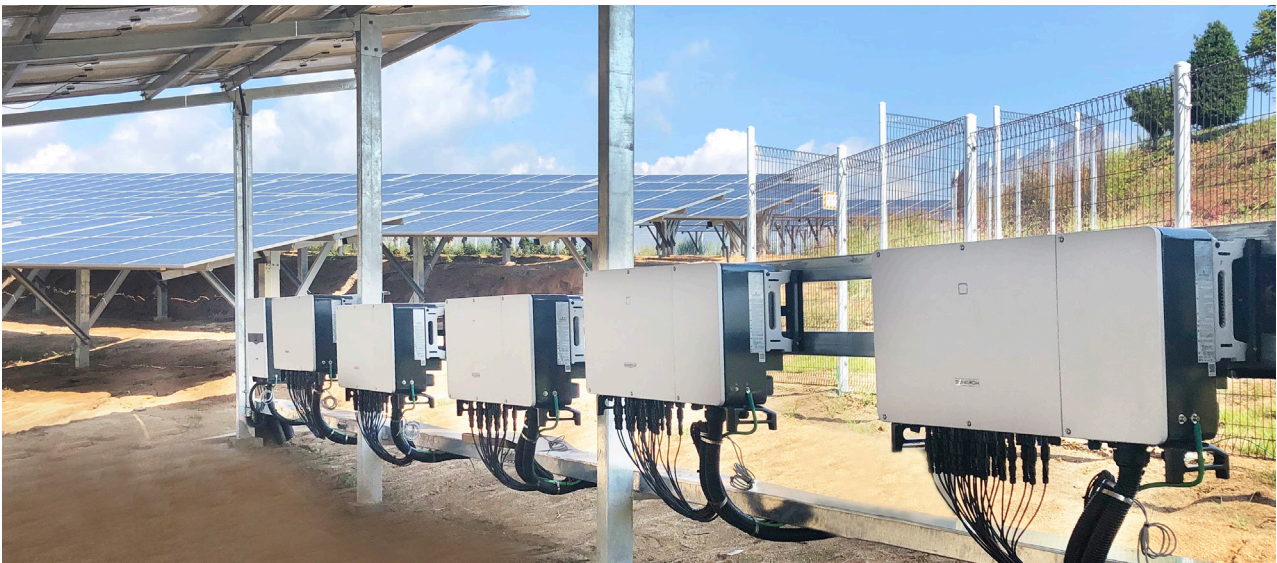
Fig.3 1MW PV Project Utilizing SG110CX in Yecheon, South Korea
