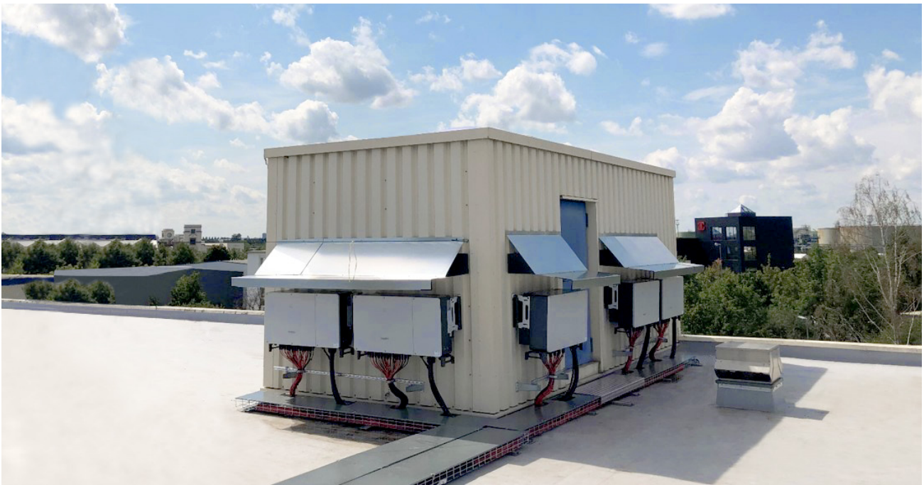
Fig.6 AC 500kW Rooftop PV Plant in Germany
