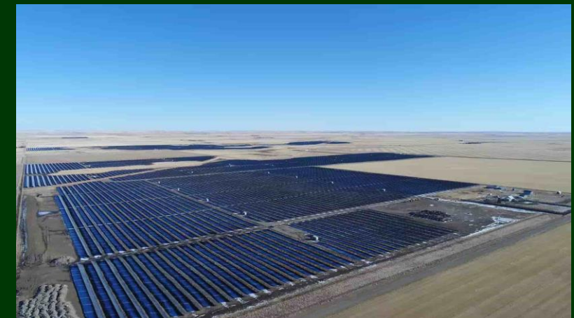
Claresholm Solar Farm, one of the Largest Solar Power Plant in Canada 132MW | Southern Alberta, Canada
