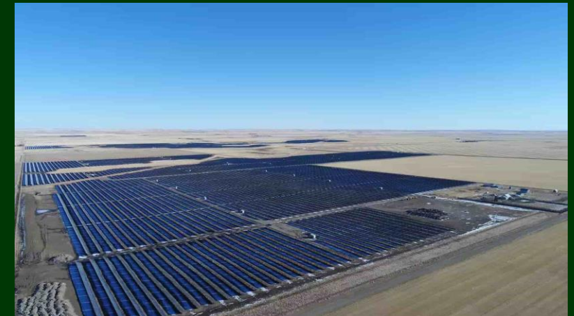
Claresholm Solar Farm, one of the Largest Solar Power Plant in Canada 132MW | Southern Alberta, Canada
