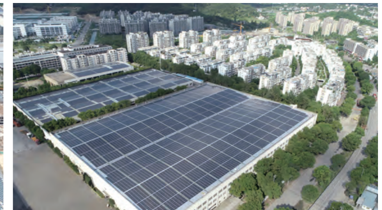
30MW Jintian Copper BIPV Power Station Ningbo, Zhejiang Province, China
