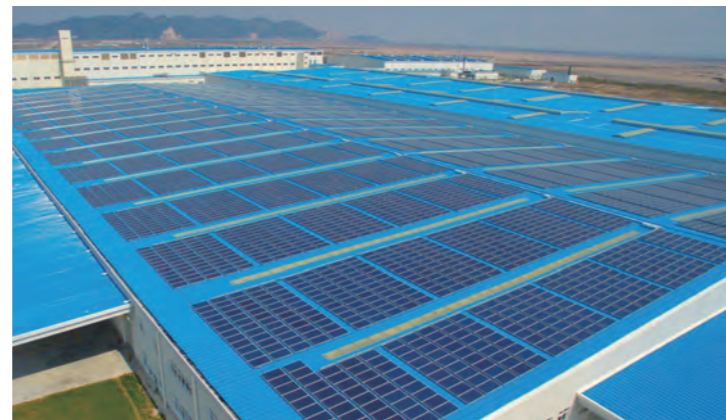
10.3MW Geely Automobile PV Rooftop Project in Linhai Linhai, Zhejiang Province, China
