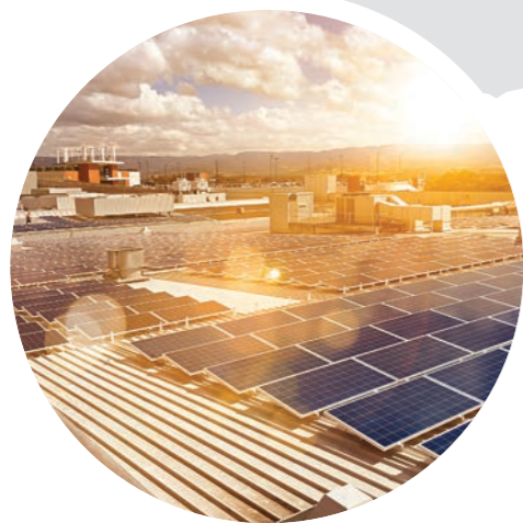
3. SHELLHARBOUR SHOPPING CENTRE, NSW Module: CS6P-P Power generation: 1.2 MW
