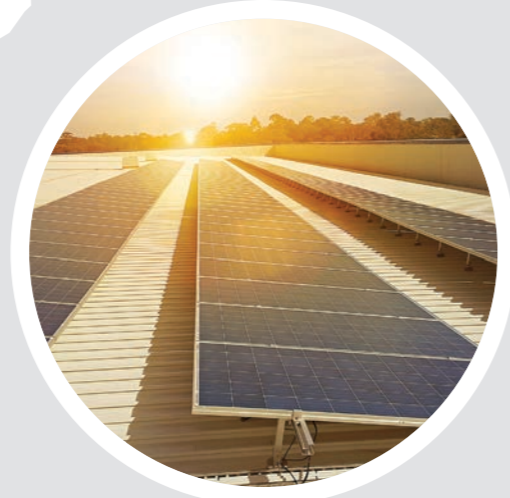
2. IKEA NATIONAL PROJECT, VIC, NSW & QLD Module: CS6X-P and CS6P-P Power generation: 3.6 MW
